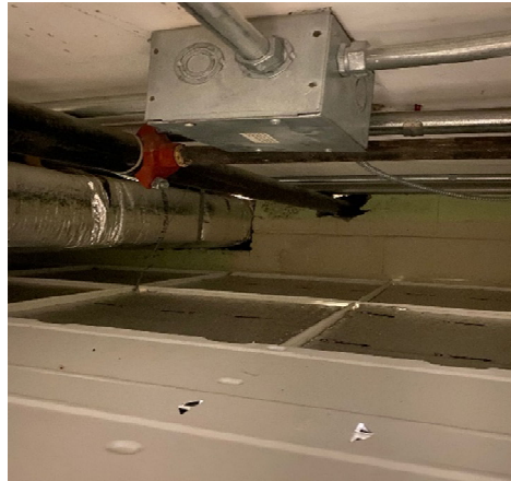
Mold on block wall/expansion joint – Lower Level
