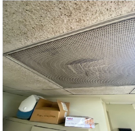
Mold Growth on Ceiling Tile – Lower Level
