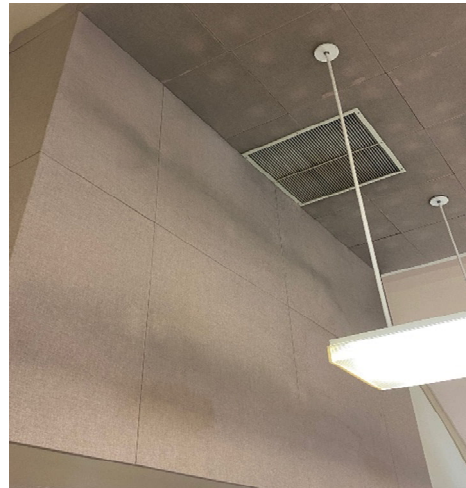
Dirt on HVAC Diffuser and Ceiling Tile – Upper Level
