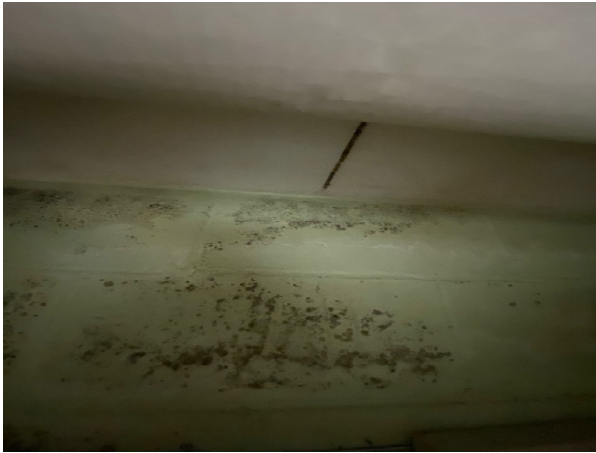
Mold on Block Wall Lower Level
