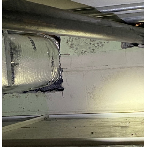
Lower Level Staff Office – Mold on Block Wall
