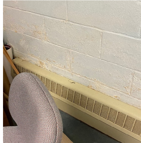
Water Intrusion Evidence – Lower Level
